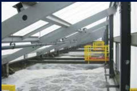
TuffSpan panels & beams at wastewater treatment plant
