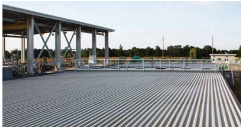
TuffSpan walk-in cover with FRP beams UV Disinfection Process
