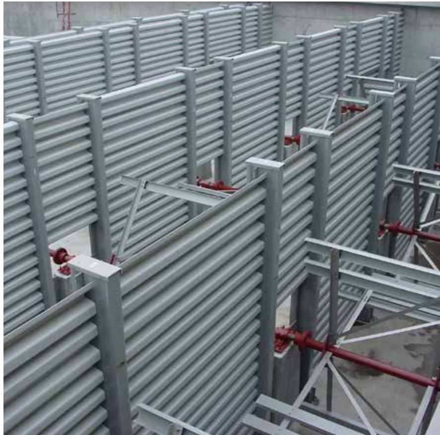
Flocculation Baffle Walls using Enduro Baffle D
