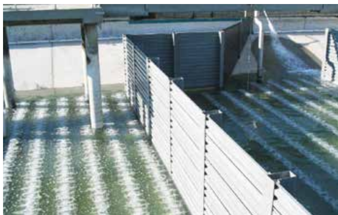
FRP SlideGuide "H" baffle series in aeration basin
