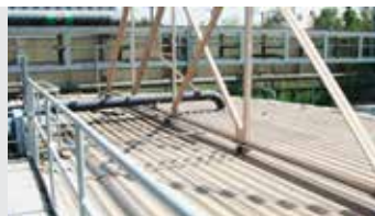
TuffSpan truss- supported cover
